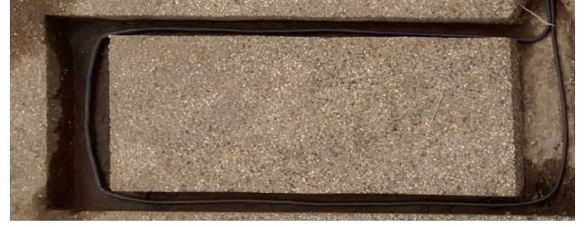
Fig. 7. Structure of the transmitter coil for system B during the embedding in the road surface.
