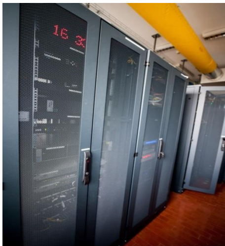
Figure 1: DEMETRA- Demonstrator assembled and integrated in the Laboratory at INRIM, Italy.
