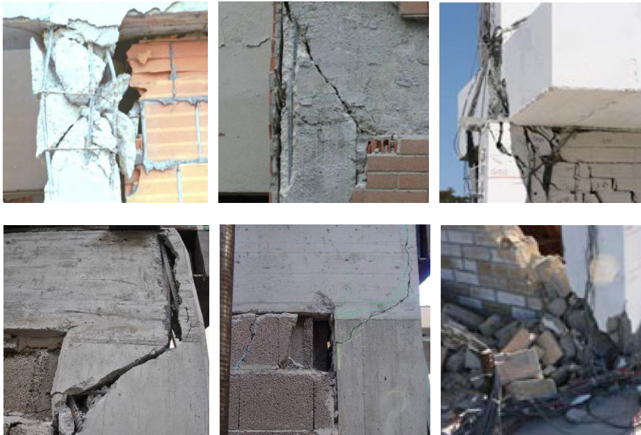
Figure 2. Local shear failures of frames due to interaction with infills under seismic loads.
