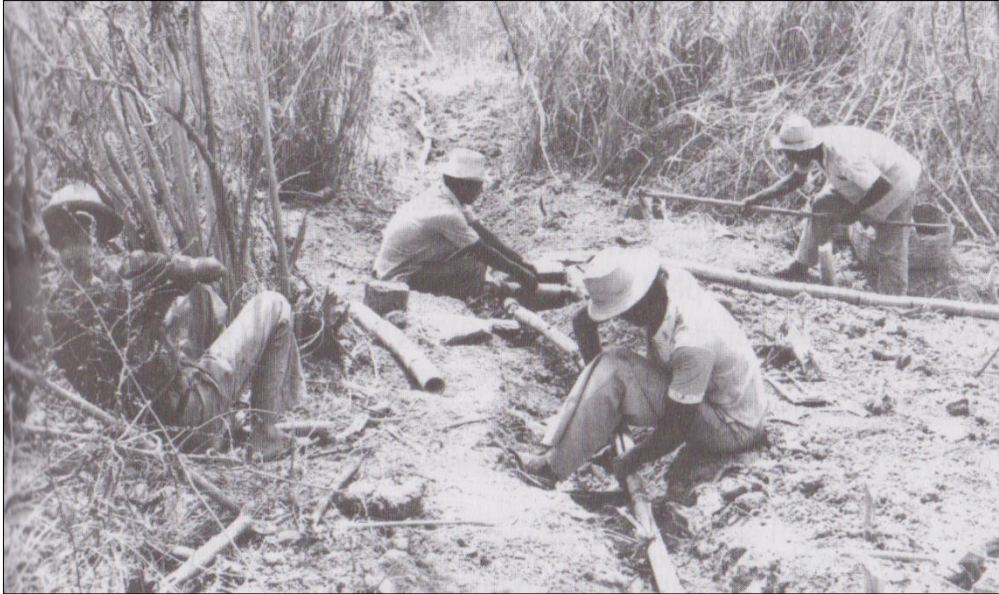
Figure 39: Construction of water supply system having bamboo as raw material - Juramento Project of Alternative Technology. In Moraes (2006).
