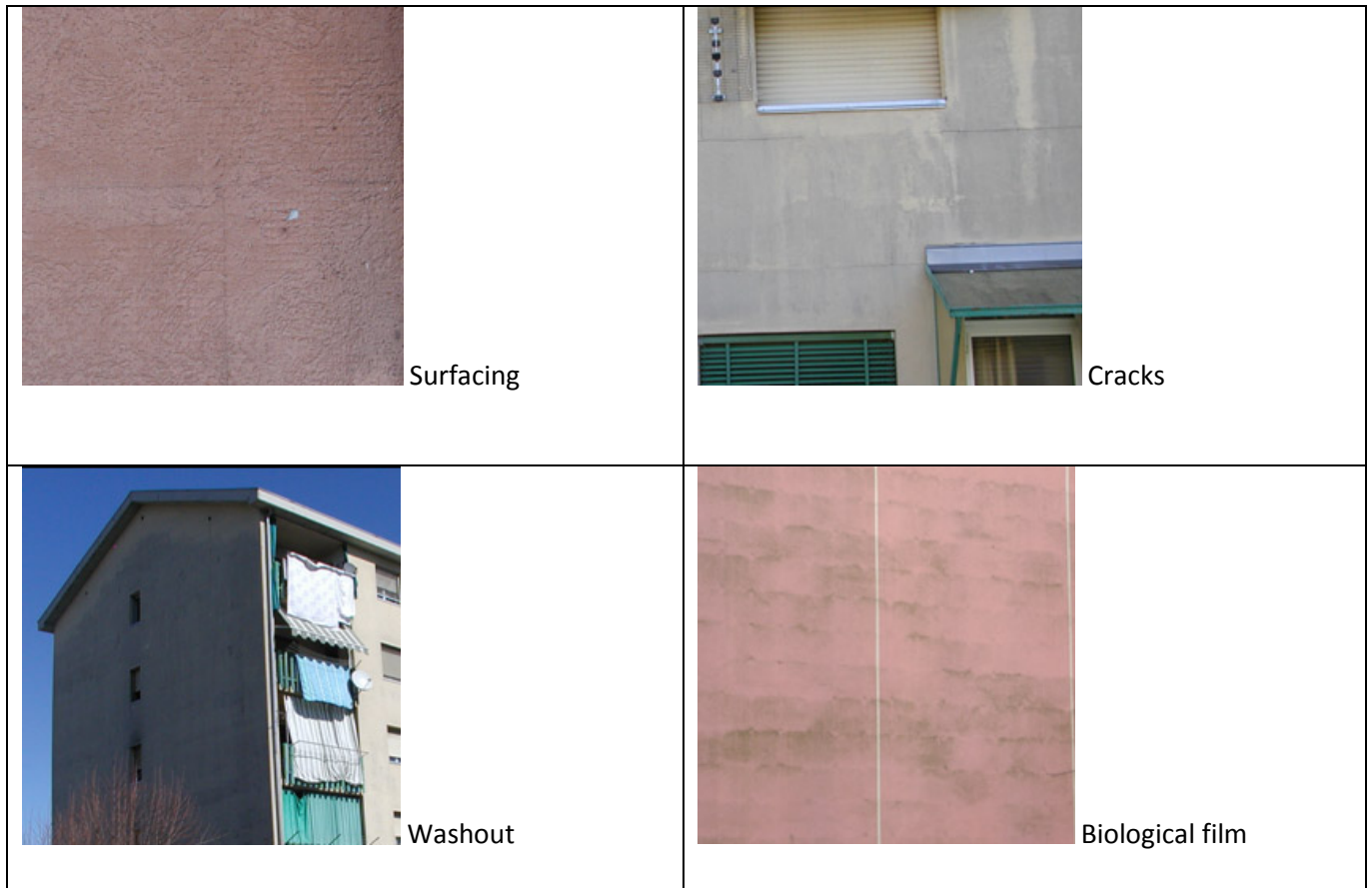
Fig 2: The main defects considered in the study.
