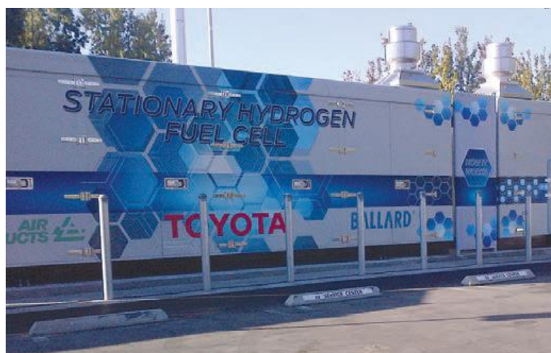
Figure 1.9. 1.1 MW PEM fuel cells Ballard system installed at the Toyota Motor Sales in USA [23].
