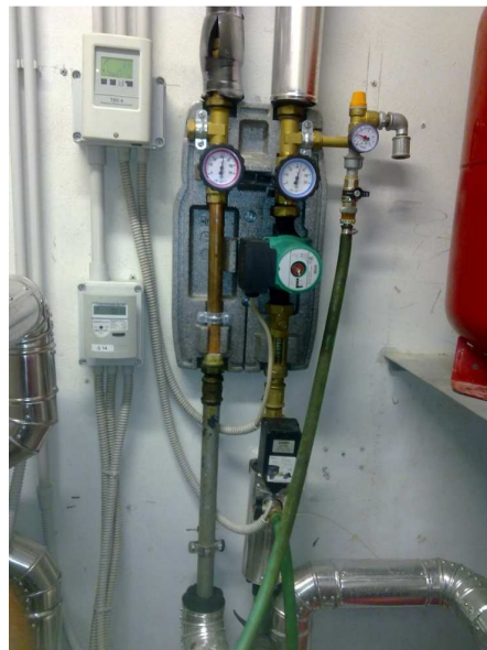
Figure 80 Solar collector circuit in PUEEL
