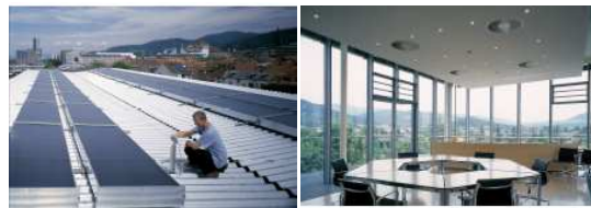
Figure 12A solar desiccant cooling system in Freiburg, Germany
