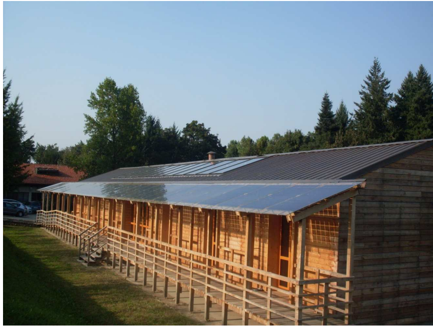
Figure 79 Solar thermal collectors and PV collectors on the roof of PUEEL building
