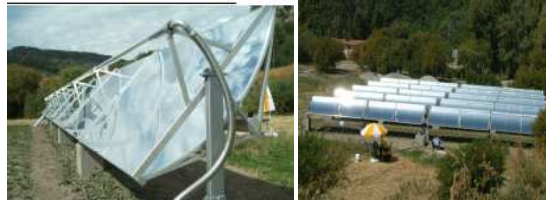
Figure 13 Air-conditioning of a hotel with parabolic trough collector in Turkey
