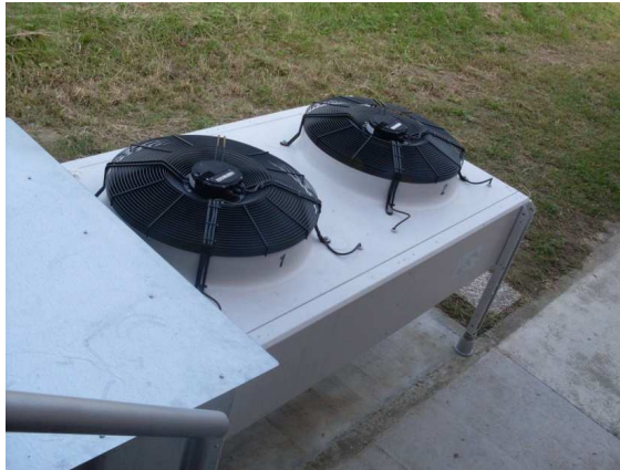
Figure 81 Dry cooler in PUEEL
