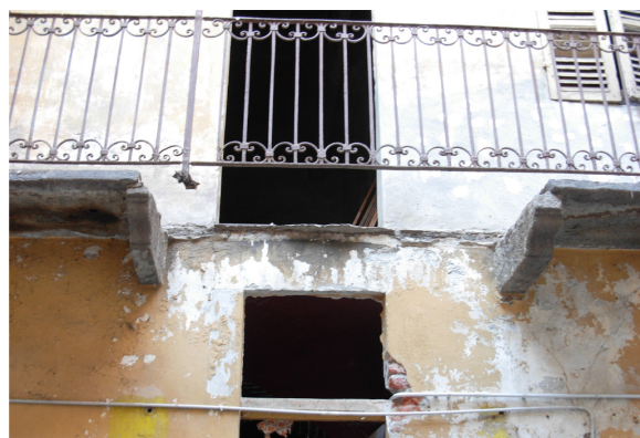
Figure 1: The remains of a balcony in Pietra di Courtil.
