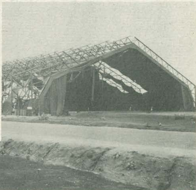
caused considerable damage to our big hangars.
