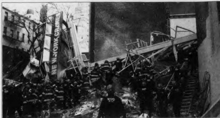
COLLAPSE: Workers in New York scramble to find missing people trapped under the rubble of a crane yesterday.
