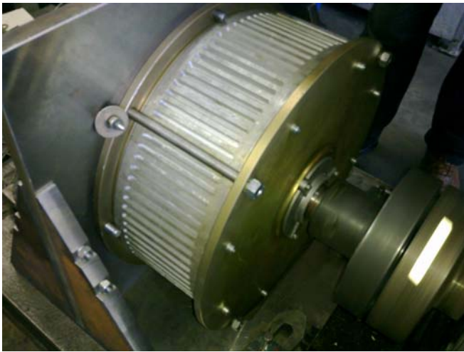
Fig. 9. Photo of the 5 KW PM generator.
