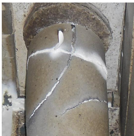
Fig. 1. Cracks on the connecting channel in the manufacture of zinc oxide. (full colour version available online)
