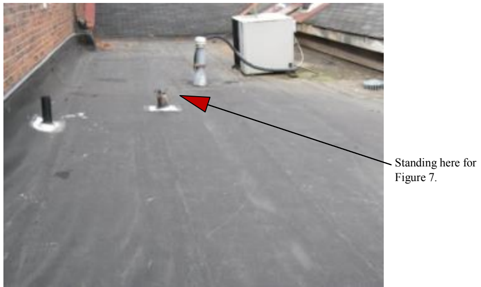
Figure 6: Garden roof location, before vegetation, as standing at the edge of the roof above the parking lot. Refer also to Figure 7.
