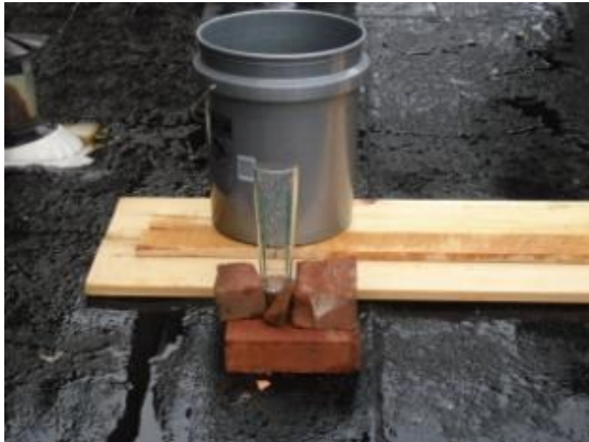
Figure 8: Rain Gauge and bucket on control roof.
