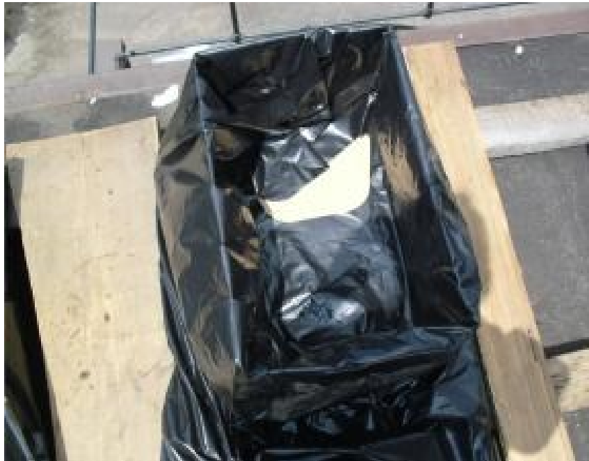
Figure 13: Interior of planting box, made by 1-bag method. Box has been placed on drainage board (not in photo) and both were placed inside the bag. The top of the bag is tucked inside the box.
