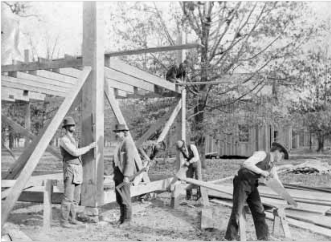
Early carpentry class. “Practical” education was very much a part of student learning in Berea’s formative period. Students often applied their learning in various building projects on campus.
