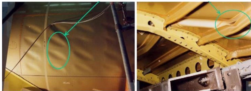
Figure 2-14: Flambage du fuselage en service.
