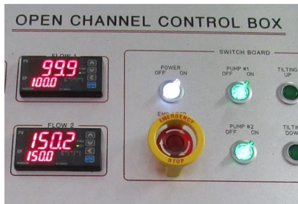
(b) Control box for pump
