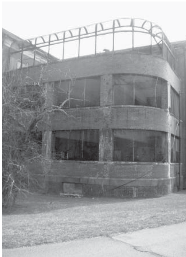
The “cages,” screened porches, on the Unit V and MR building. This building was at one time the tuberculosis unit. (Photo in 2008)
