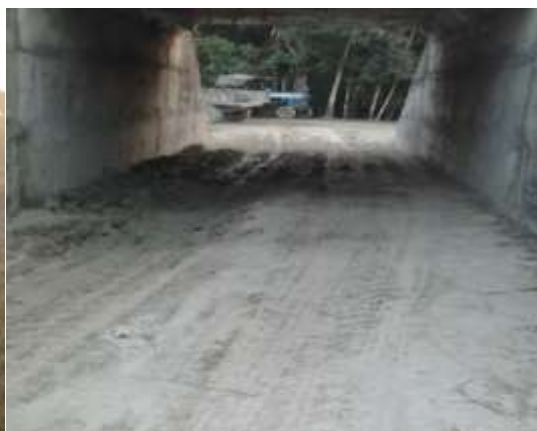
Plate-2: Showing the road condition due to transportation of soil.
