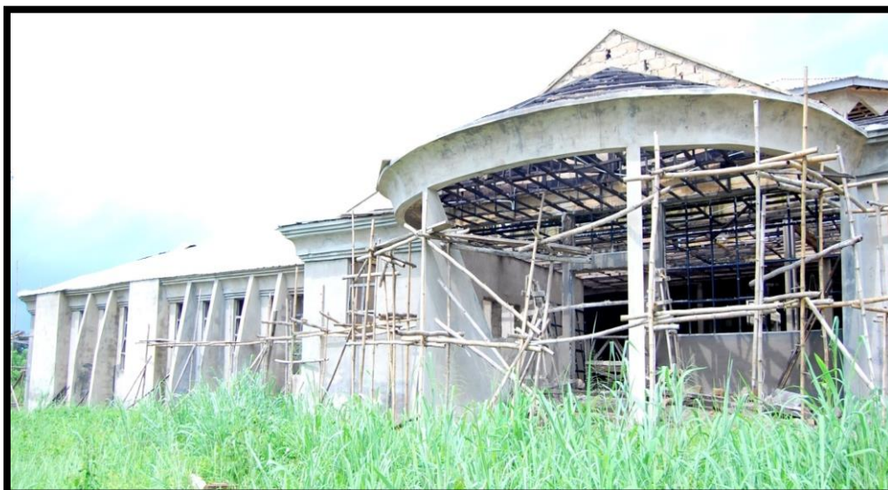
Pictures Showing the Construction of the new library building across the six campuses, projected beyond Vision 2030.
