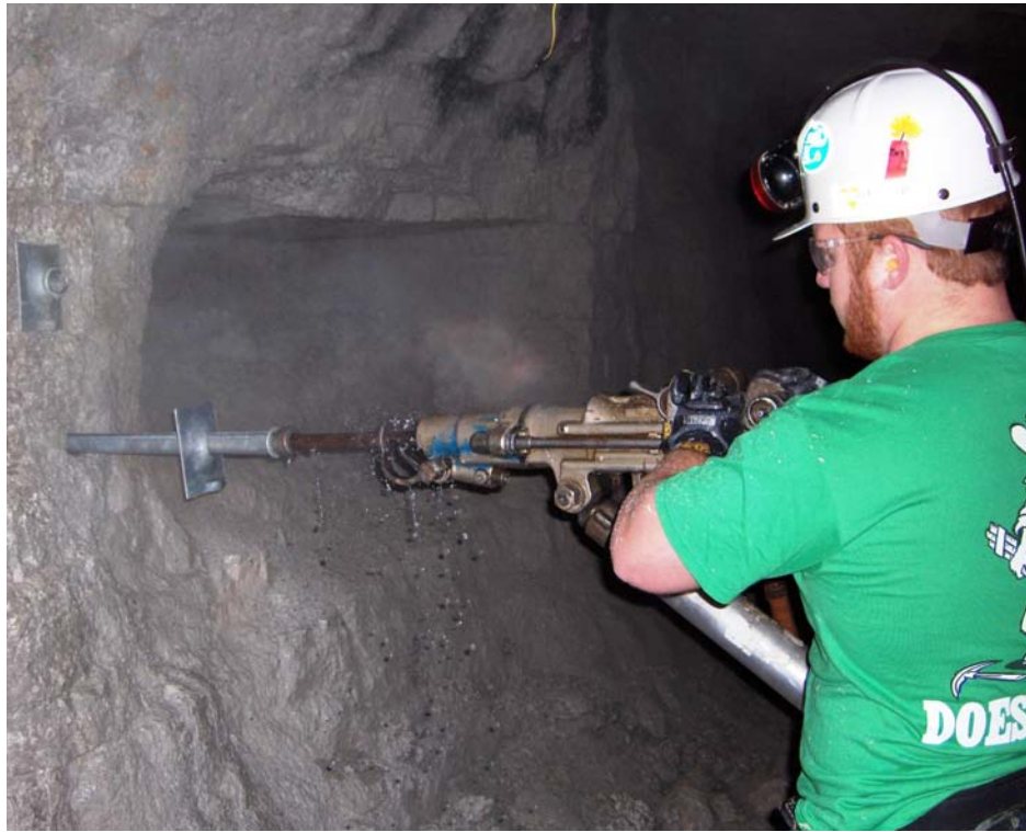
Figure 4.20. A Participant Installing a Split Set Rockbolt During the Underground Rockbolting Contest.
