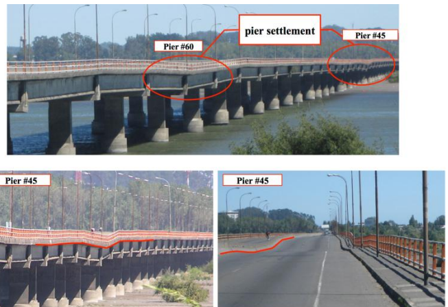
Fig. 8. Liquefaction-induced vertical settlement along the Juan Pablo II Bridge.
