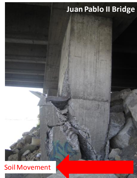
Fig. 9. Failed pier at the north end of the Juan Pablo II Bridge.
