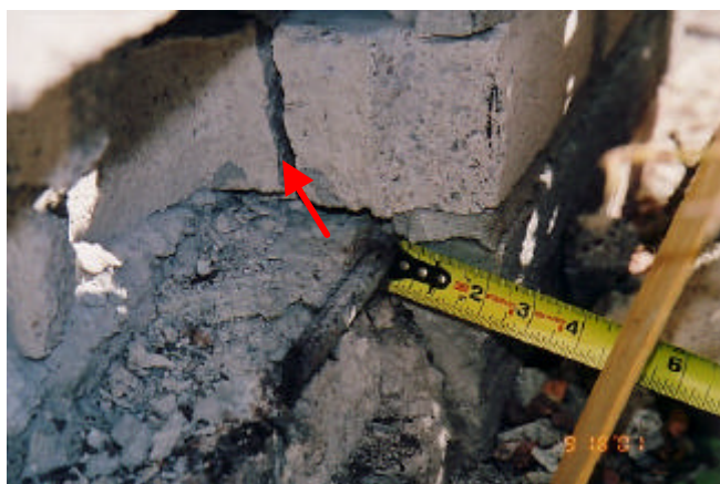
Fig. 5. Example showing existence of vertical crack in the central portion of a wall. The arrow points to the outer face of the block wall.
