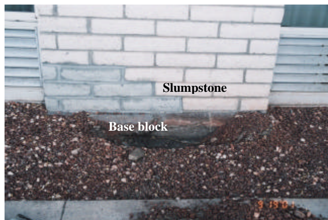
Fig. 2. Typical narrow exterior wall. Note that previous destructive testing had been performed on the left side of the wall.
