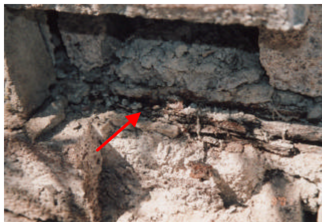
Fig. 7. Example of severe corrosion of reinforcement in concrete. The arrow points to corrosion product as the original steel was completely corroded.
