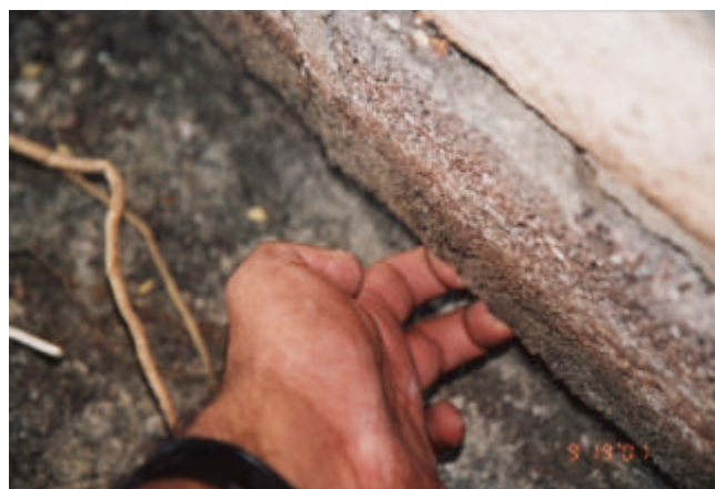
Fig. 6. Typical cracking of base block. This condition was observed around the entire perimeter.
