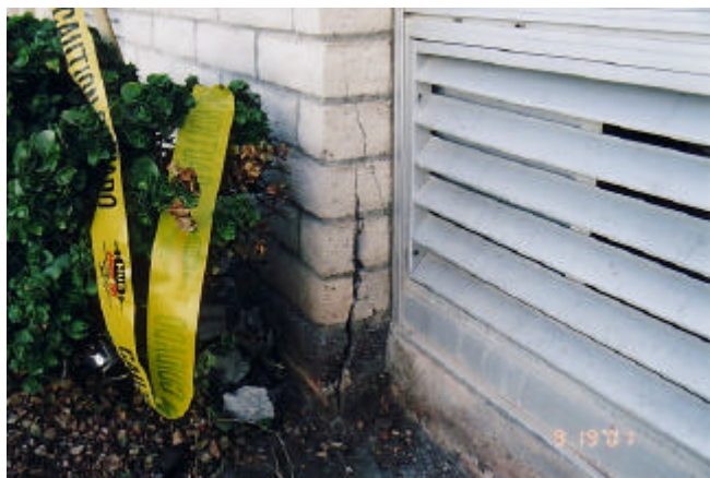
Fig 4. Typical damage observed at base of slender CMU wall.
