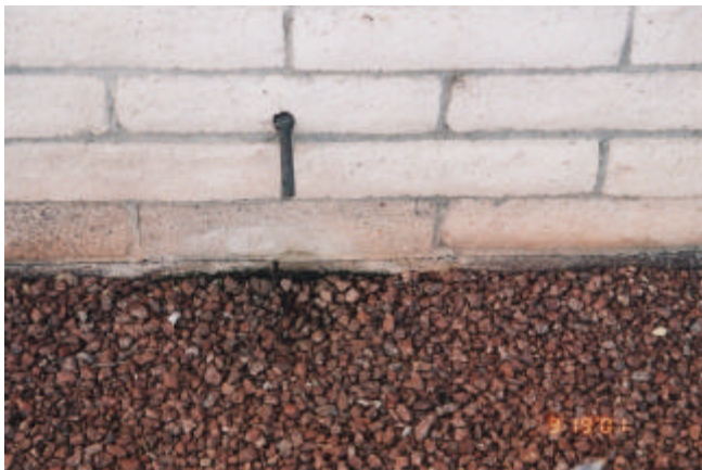
Fig. 13. Example of deteriorated concrete located next to a source of water.
