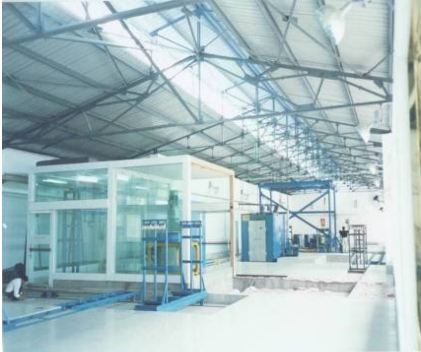
The 1st production line of self-cleaning glass based on \text{TiO}_2 films in China found in August, 2002
