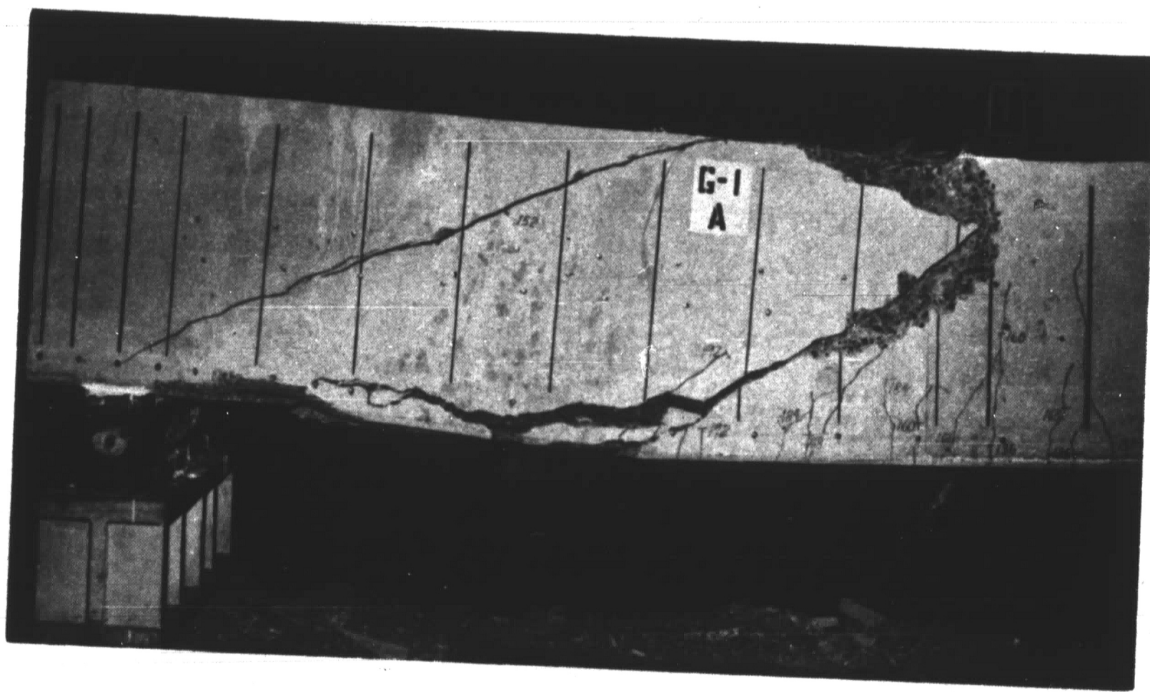
b. Left Side of A Shear Span After Torsional Inclined Cracking and Failure
