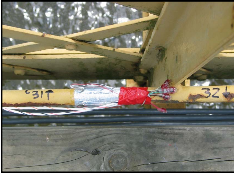
Figure 4.11 – CH_31 and CH_32 installed on the east and west faces, respectively, of the diagonal tension bar, which ties the east Z-Bar arch near floorbeam 2 to the bottom end of the vertical T-shape member at floorbeam 8. The gages were installed at a diagonal distance of approximately 11'-6" away from the end of the bar at floorbeam 8.
