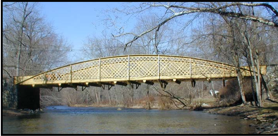
Figure 1.1 – Elevation view of the Hares Hill Road Bridge over French Creek (View looking west)
