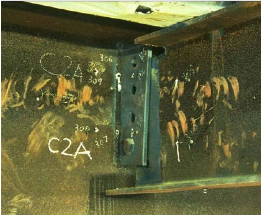
Figure 2.21 Failure of the fin-plate on the shear tab connection in British Steel Test 2 (Newman, 2000)
