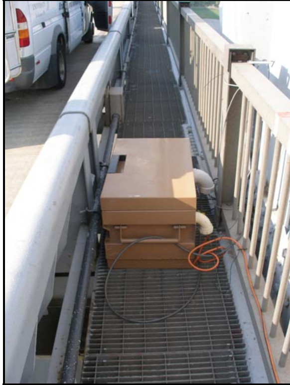
Figure 2.2 – Weather-tight box containing data acquisition system located on the west-bound walkway at Panel Point 6
