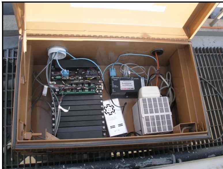
Figure 2.3 – Interior of weather-tight box containing data acquisition system
