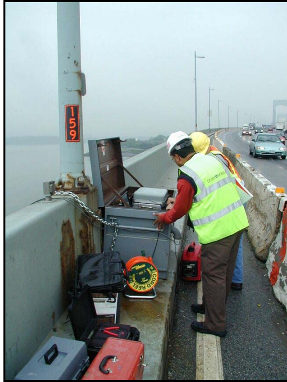
Figure 3.2 – Weather-tight enclosure containing data logger and batteries
