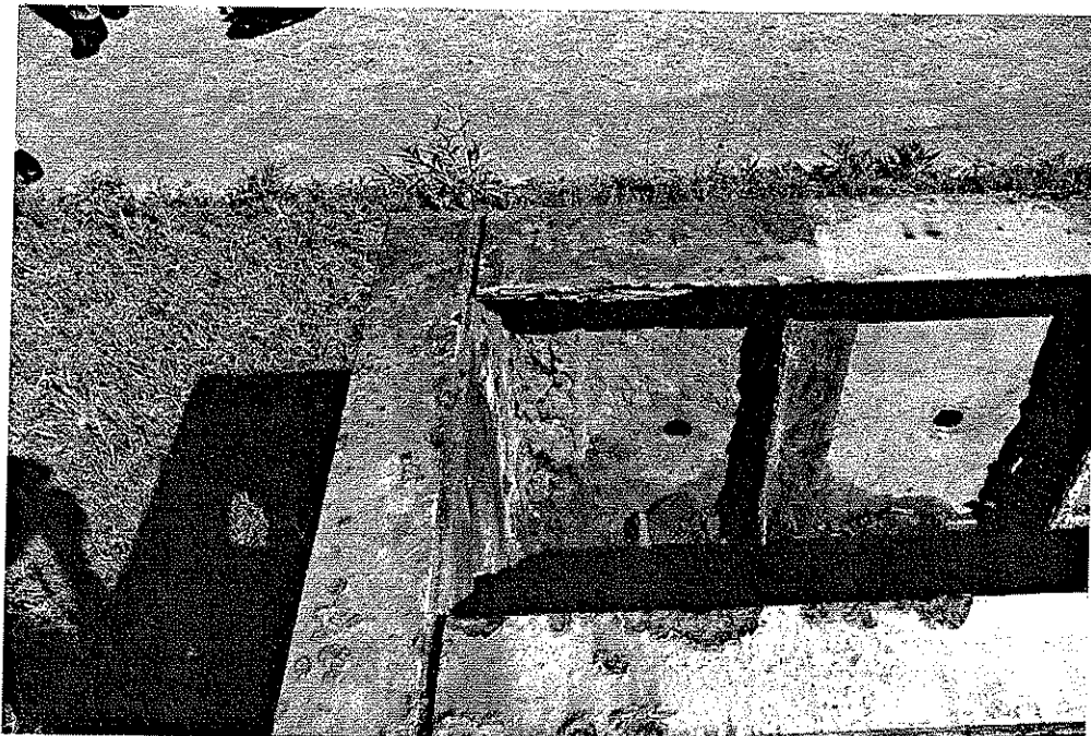
Figure 13: Heavy Corrosion in Lower Corner of Lift Gate at Bankhead Dam (5/92/1-8)
