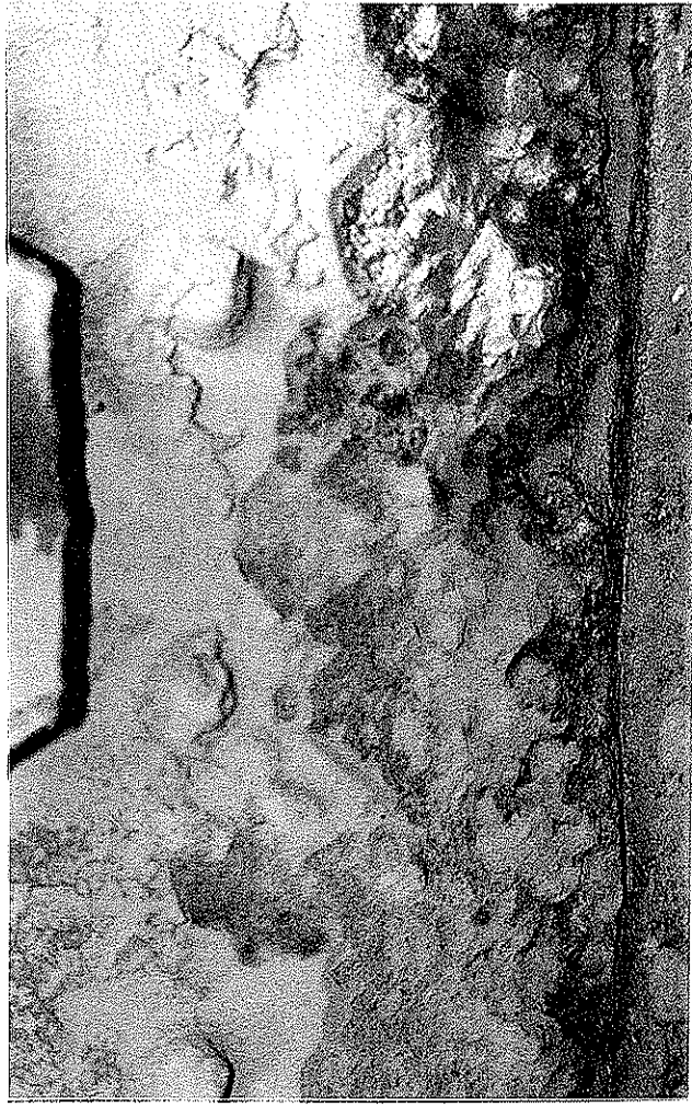
b) Closeup of section loss in region of D26 (1/98/8-21)
