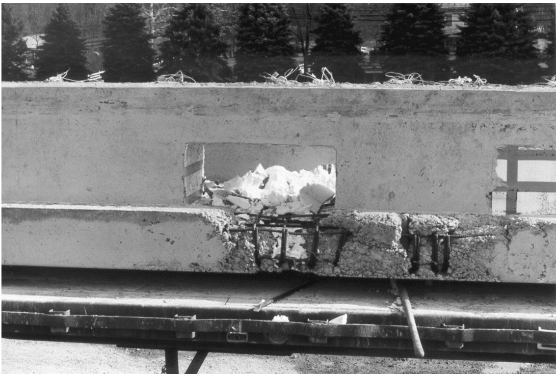
Figure 2.11 S3 at midspan showing lack of consolidation at midspan
