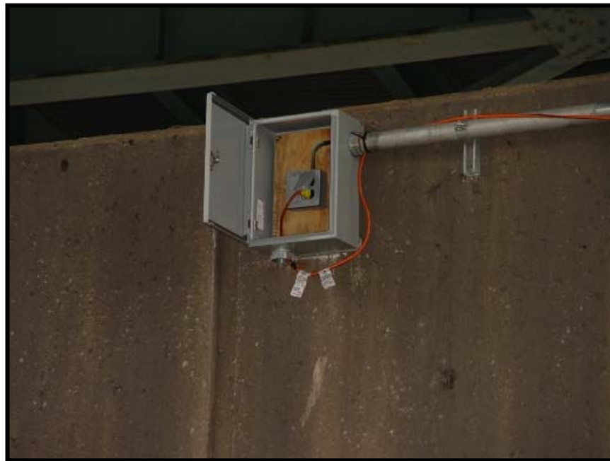
Figure 2.3 – Power supply junction box on pier 11
