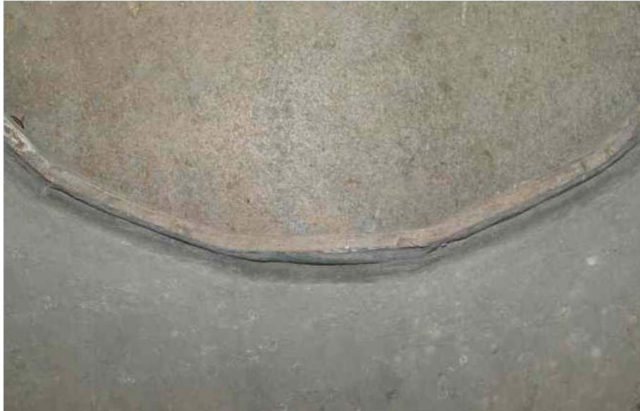
Figure 2.3 – Close-up view of cracked weld in baseplate
