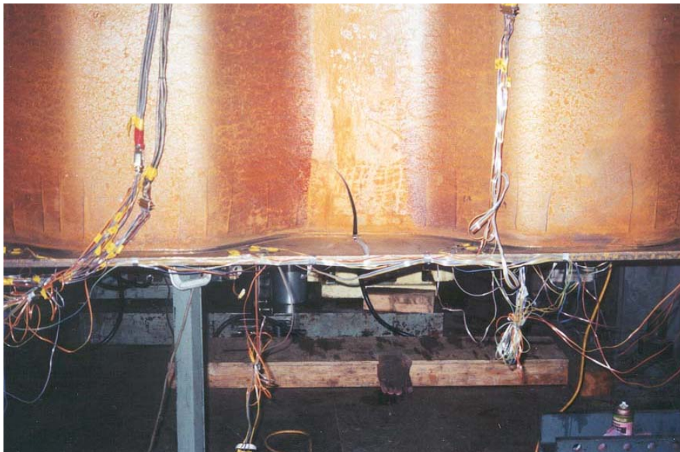
Figure 24. Failure of Girder G1B.
