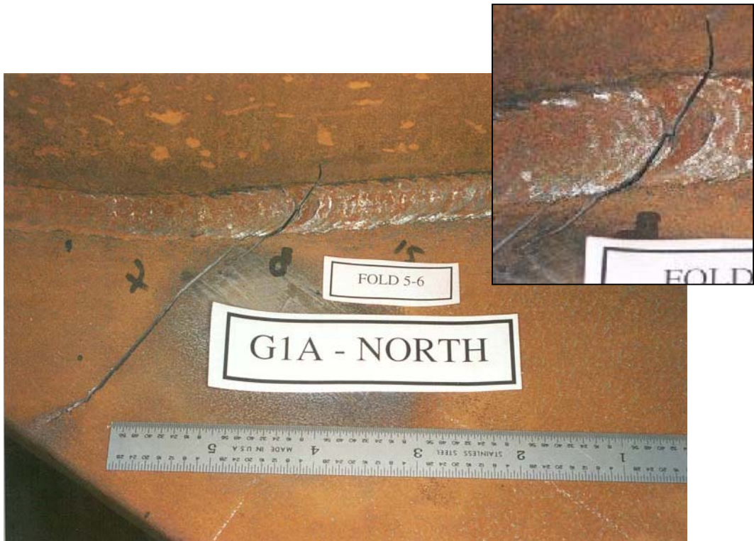
Figure 18. Main fatigue crack of Girder G1A.
