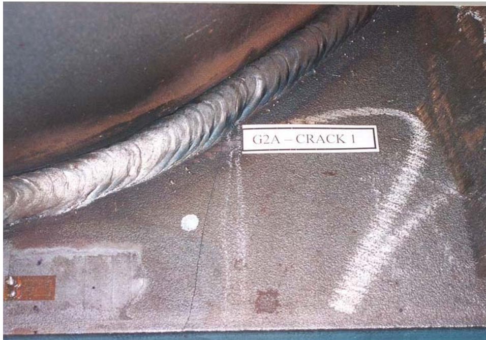
Figure 17. Main fatigue crack of Girder G2A.
