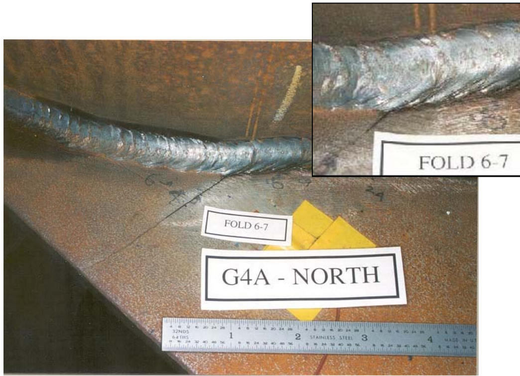
Figure 19. Main fatigue crack of Girder G4A.
