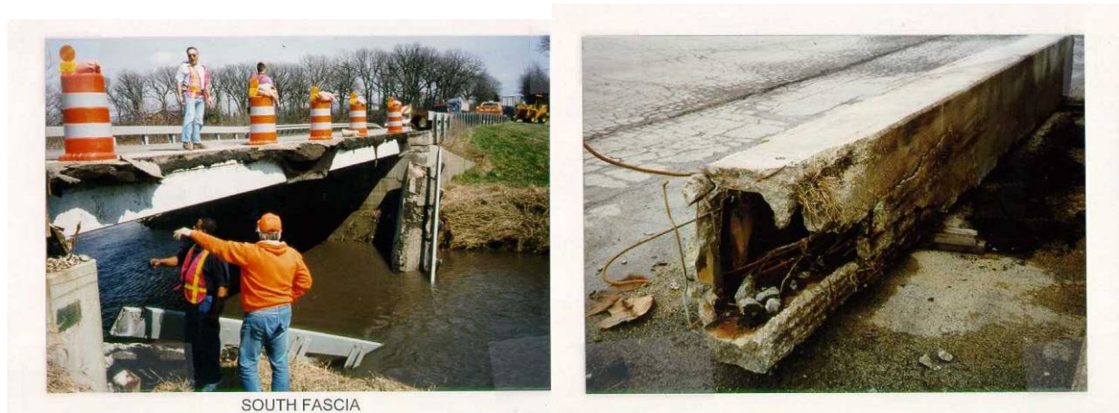
Figure 5: IDOT Structure 046-0055 Beam Failure [046-0055.ppt]
