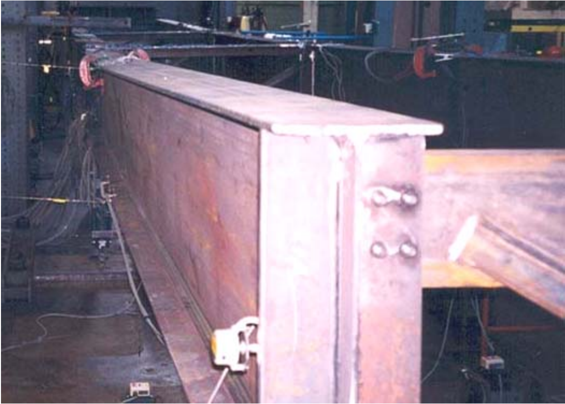
Figure 21. Photograph of north girder at peak load.
