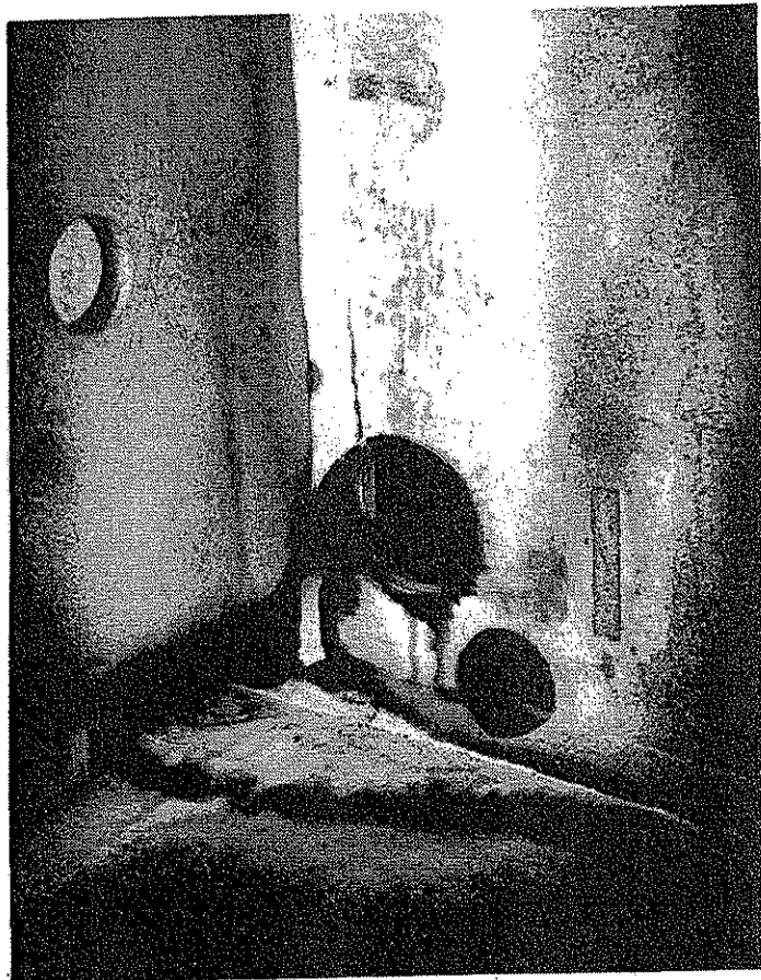
Fig. 30: Retrofitted distortion cracks at detail 1N09.
