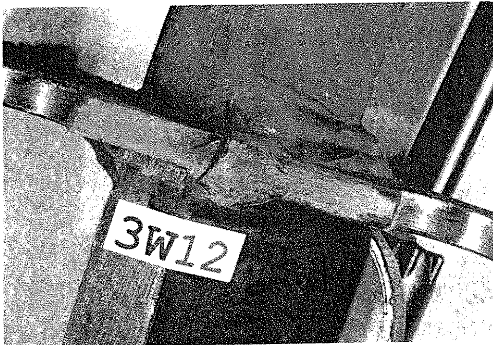
Fig. 14: Typical through thickness crack arrested by retrofit holes.
