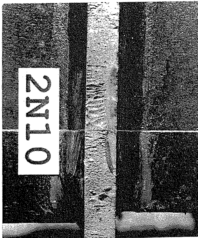
Fig. 25: Fatigue crack at detail 10, girder 2N.
