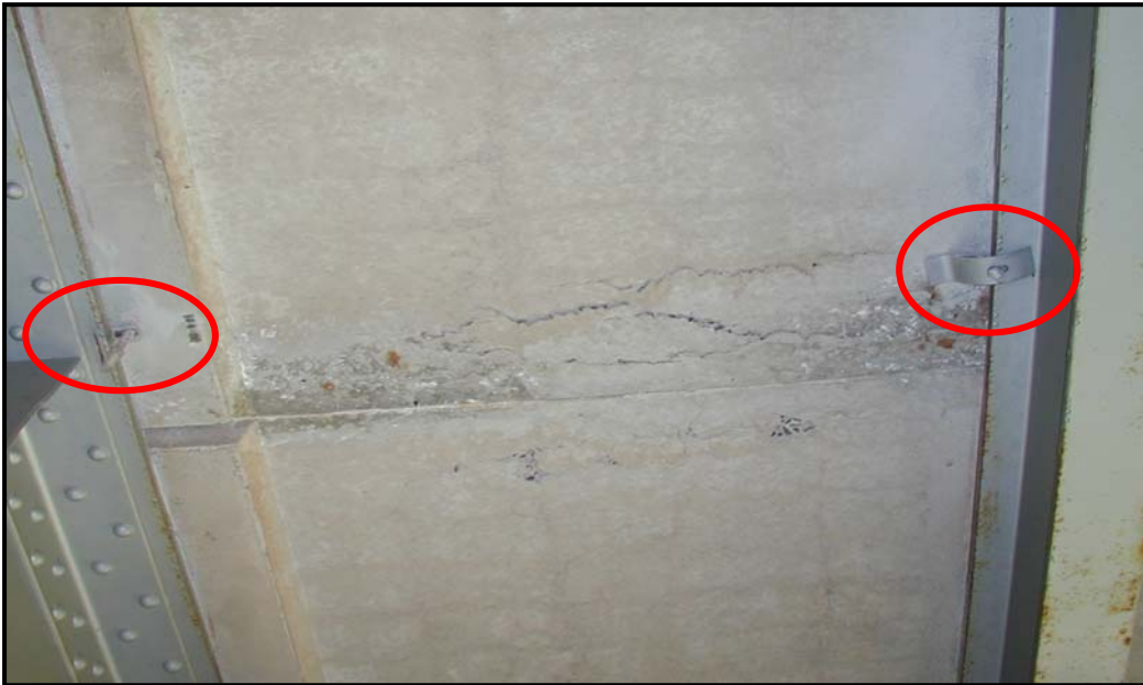
Figure 17 – Portion of bottom of deck. Notice missing spring clamp on left
