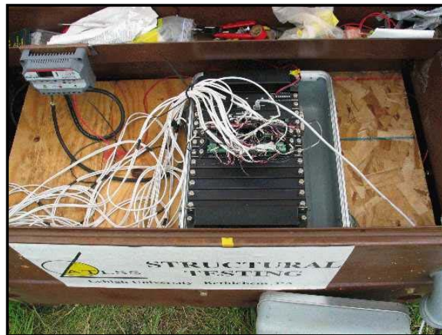
Figure 9 – Photographs of CR9000 data logger installed in weather-tight box
