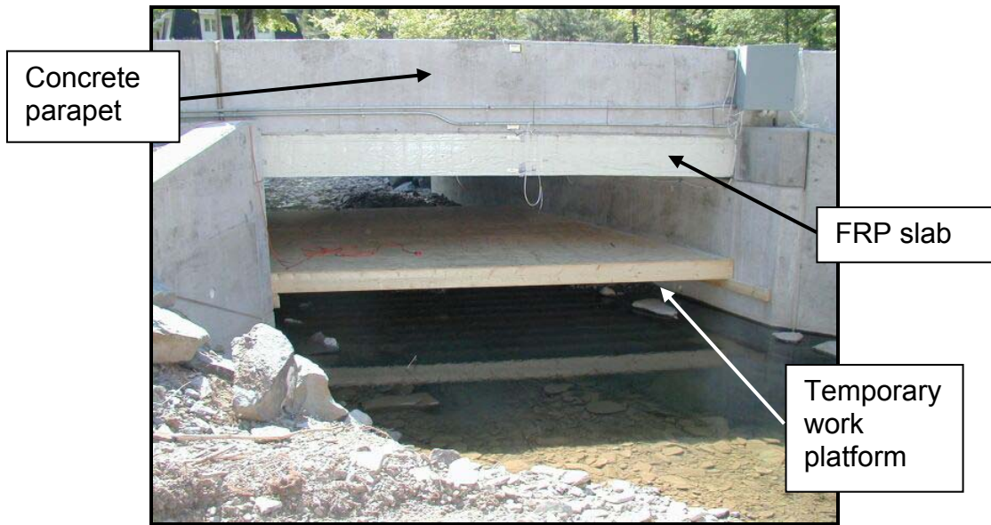
Figure 1.1 – Photograph of FRP bridge over Dubois Creek in Great Bend Twp., PA
