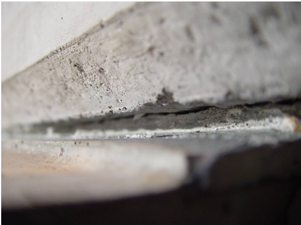
Figure 9-26: Failure of the Composite Interface
