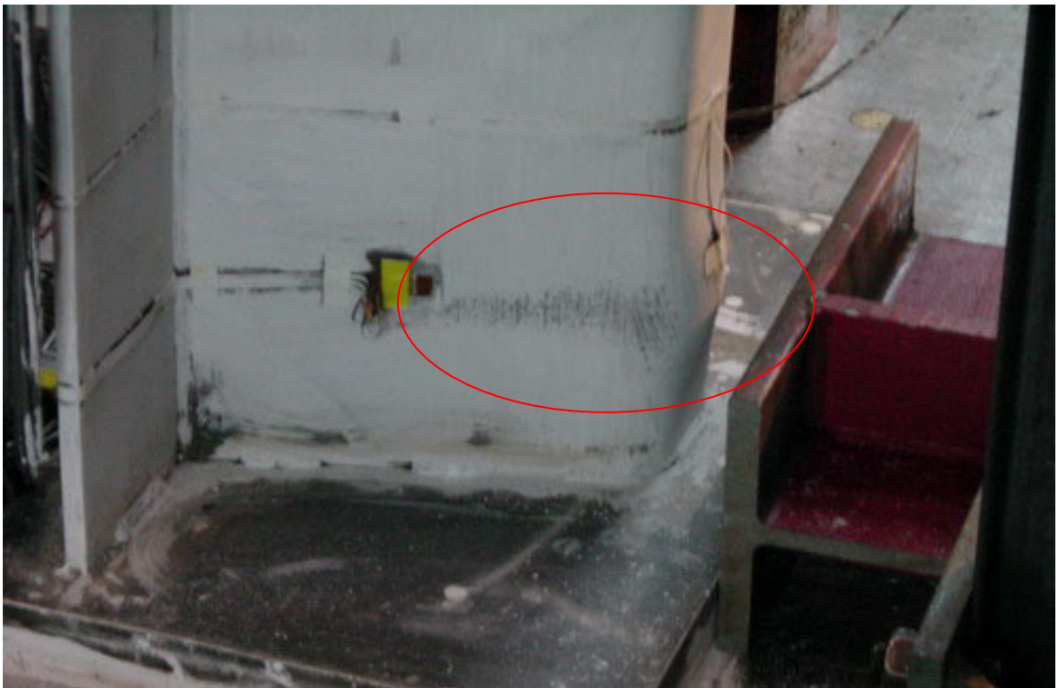
Figure 4-18 Local Buckling of Rib Wall near the Ends of Beam-column, SBC1
