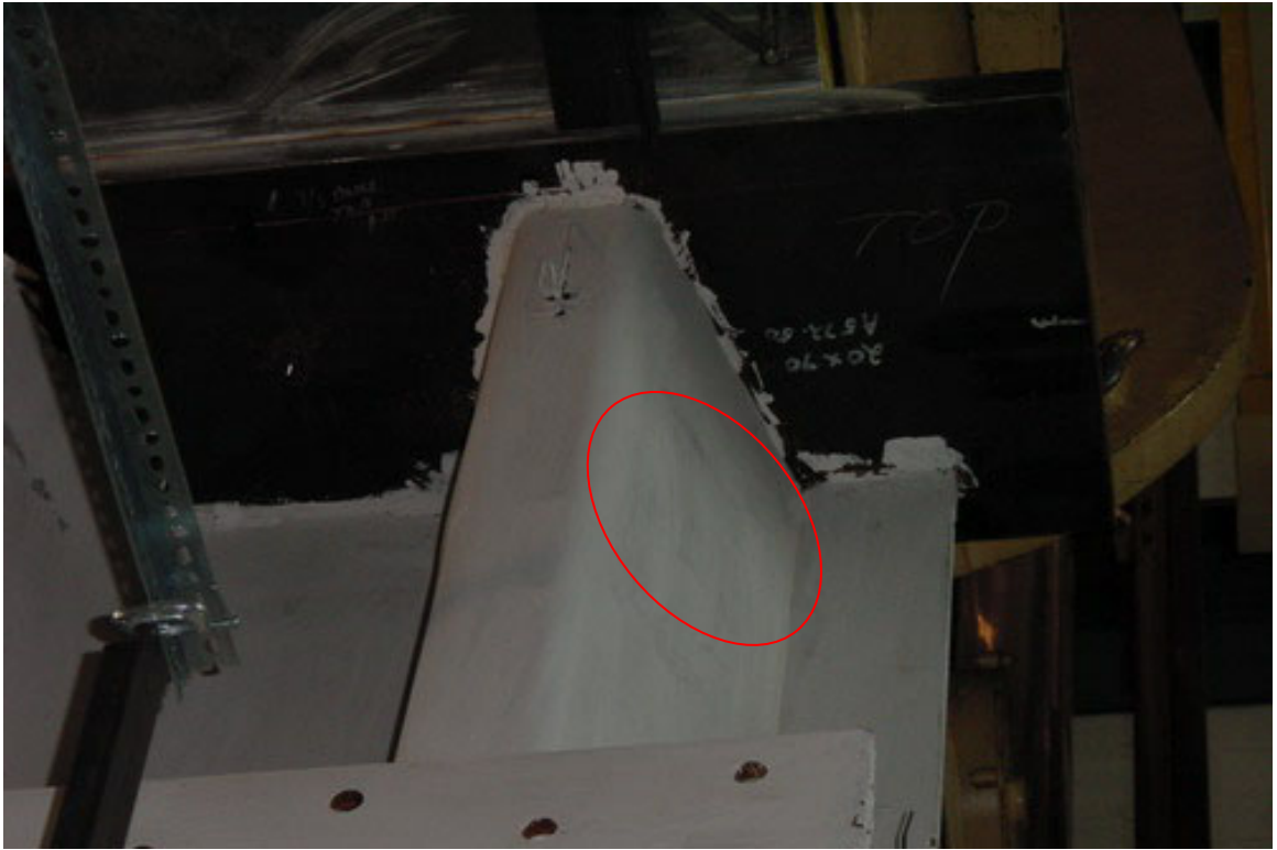
Figure 4-23 Local Buckling of Rib Wall of Triple-rib Beam-column, TBC
