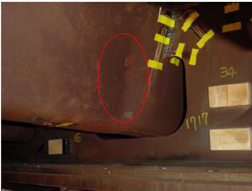
Figure 3-9 Closed Up View of Buckled Rib Wall of Triple-rib Beam
