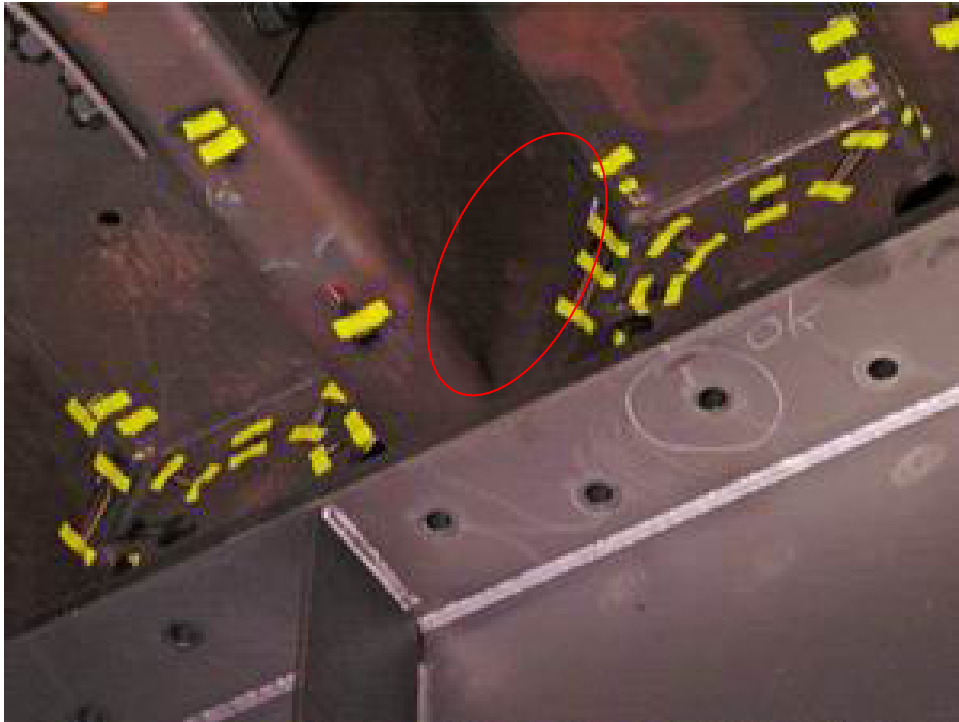
Figure 3-8 Buckled rib wall, Triple-rib Beam
