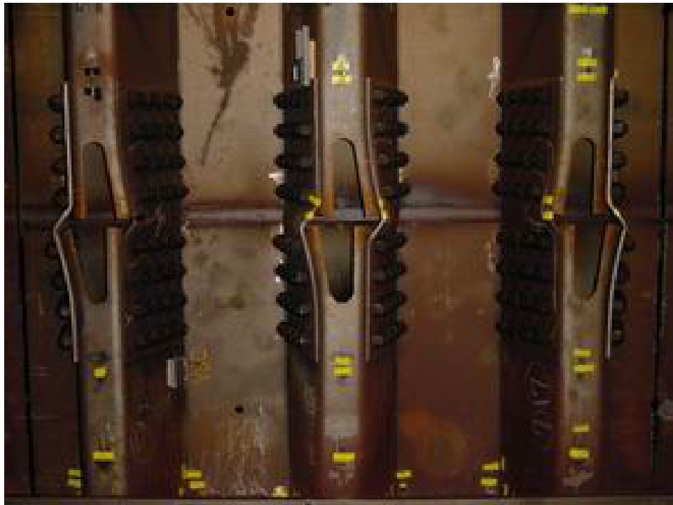
Figure 3-7 Buckled Splice Plates, Triple-rib Beam
