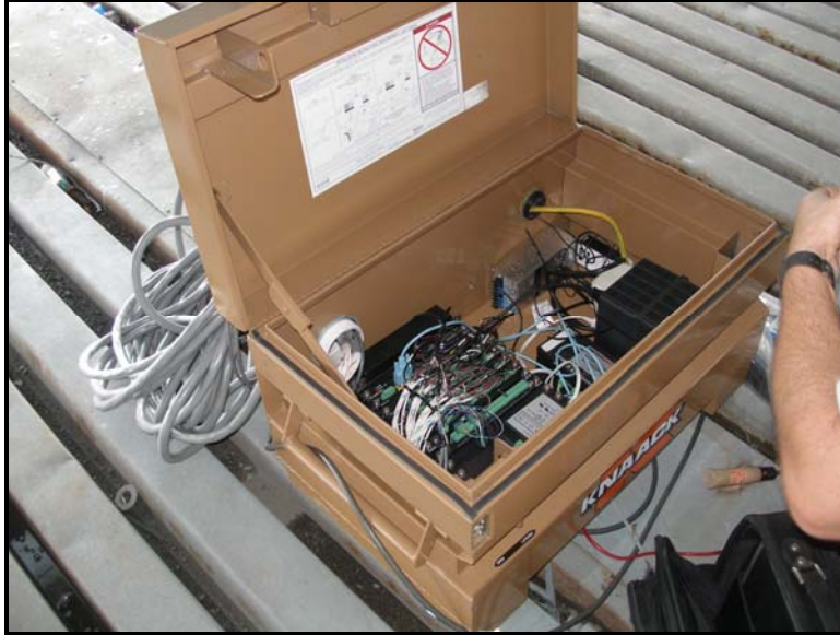
Figure 3.5 – Weather-tight enclosure used to house the data acquisition system and wireless communications
