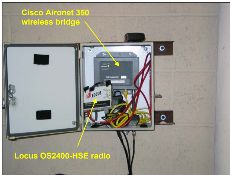
Figure 3.25: Wireless bridge and radio installed on roof of Martin Tower
