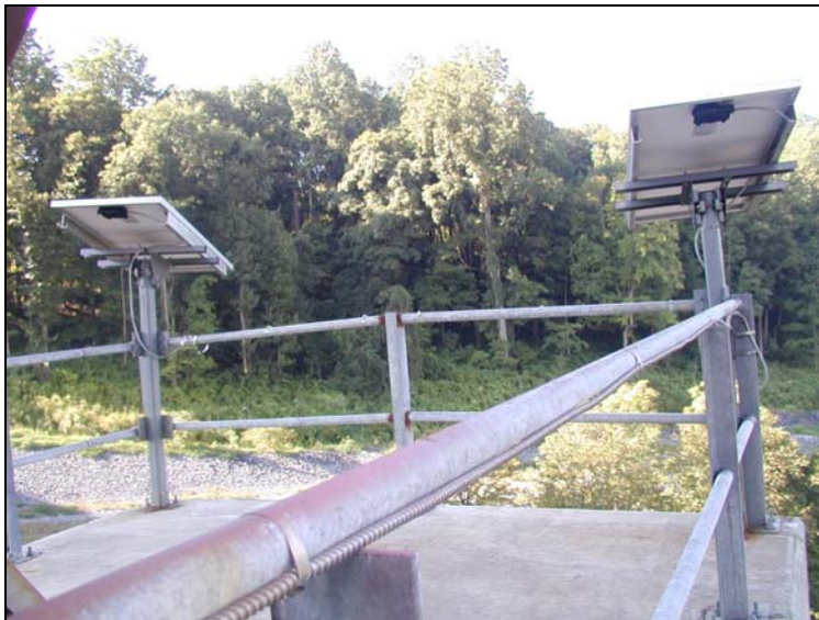
Figure 3.20: View of solar panels on pier 2 looking west
