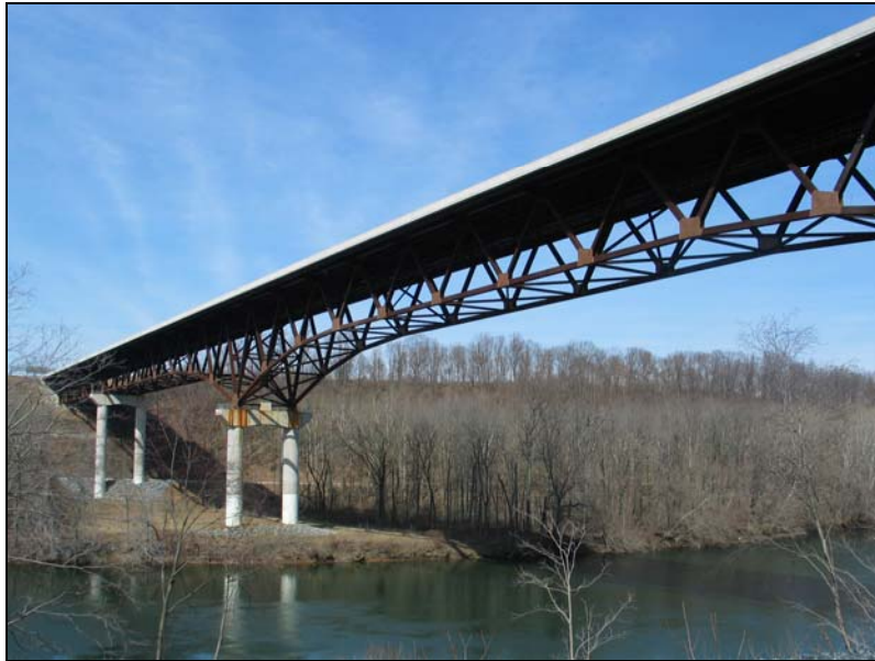
Figure 1.1: Photograph of the SR-33 Lehigh River Bridge looking northeast at the west face of the bridge
