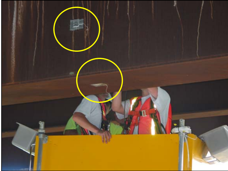
Figure 3.16: Instrumentation of the east upper chord (U26-U28 East)
