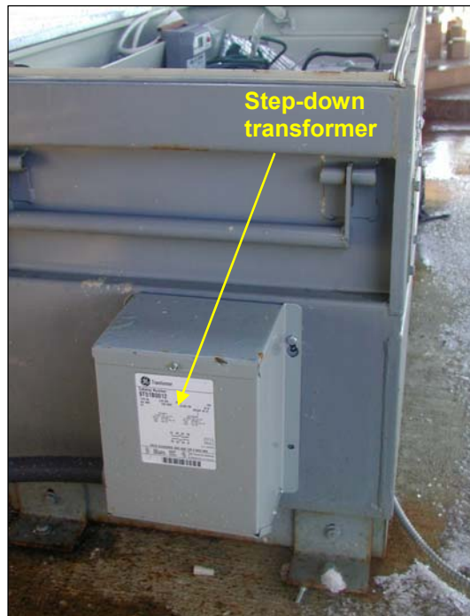
Figure 3.22: Step-down transformer mounted on east face of battery box
