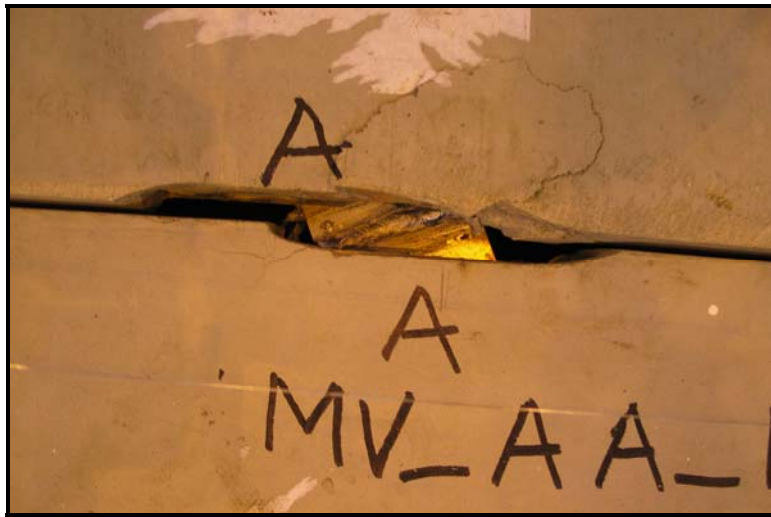
Figure 34: Specimen MV_AA-1 - condition of A-A connector at a shear load of 10.5 kips showing spalling of concrete
