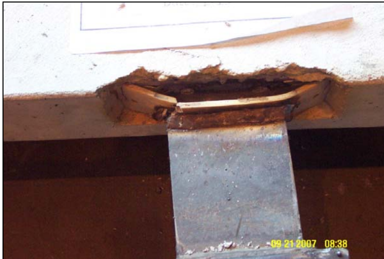
Figure 87: Connector plate fracture
