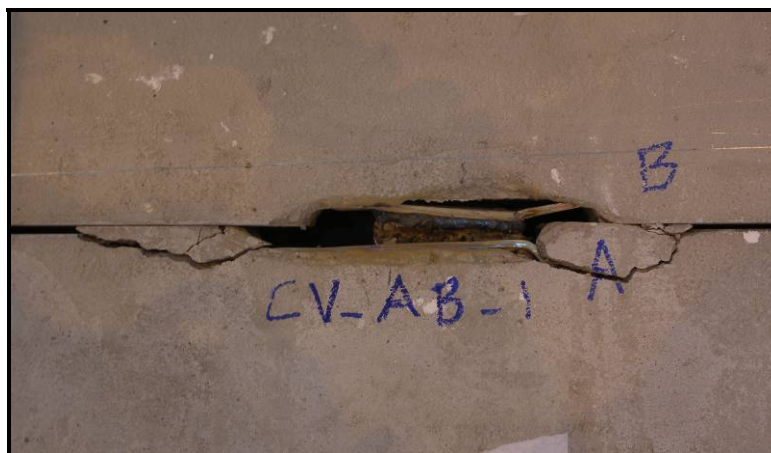
Figure 43: Specimen CV_AB-1 - spalling of top surface of panel at a load of 8.9 kips
