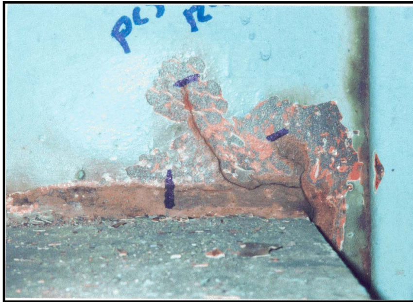
Figure 1.2 – Typical cracking of floorbeam-to-kneebrace connection
