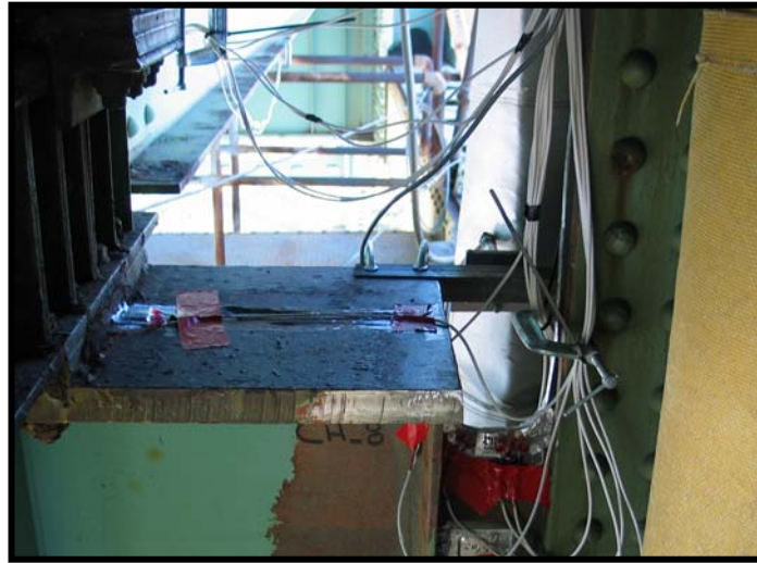
Figure 4.1 - Initial retrofit scheme at FB78 with the knee-brace removed and the cutout introduced in the web of FB78 (View looking south)
