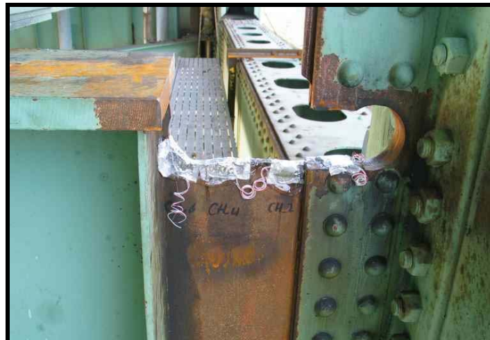
Figure 4.2 – Second retrofit scheme with knee-brace removed and the cutout introduced in the web of floorbeam FB78 as well as the back-to-back angle (View looking south)
