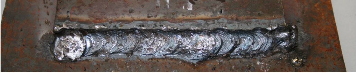
Figure 3.14: Example of Weld Classified as “Poor” (2)
