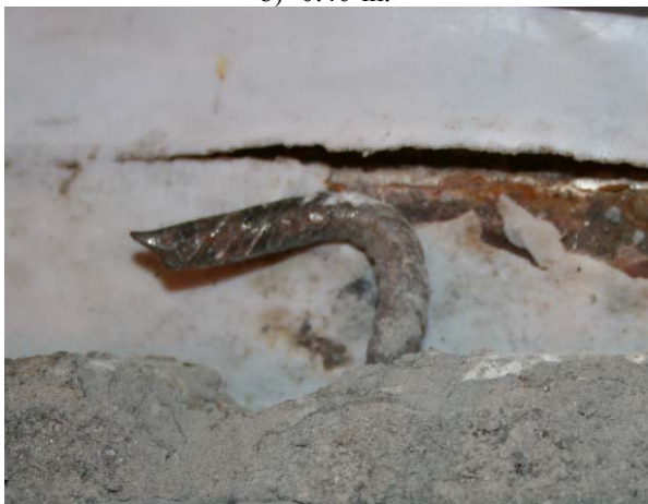
d) -2.90-in.(visible hairpin damage)
