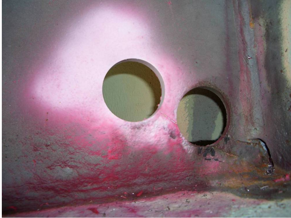
Figure 14 Holes drilled at crack tips
