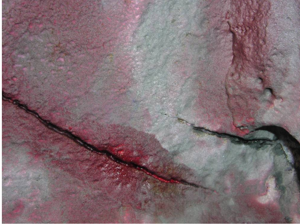
Figure 12 Crack origin (north side of bearing stiffener)
