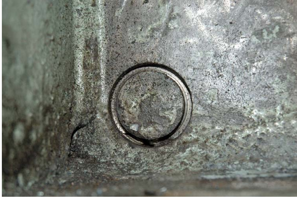
Figure 51 Attempt of drilling core to retrieve possible crack origin
