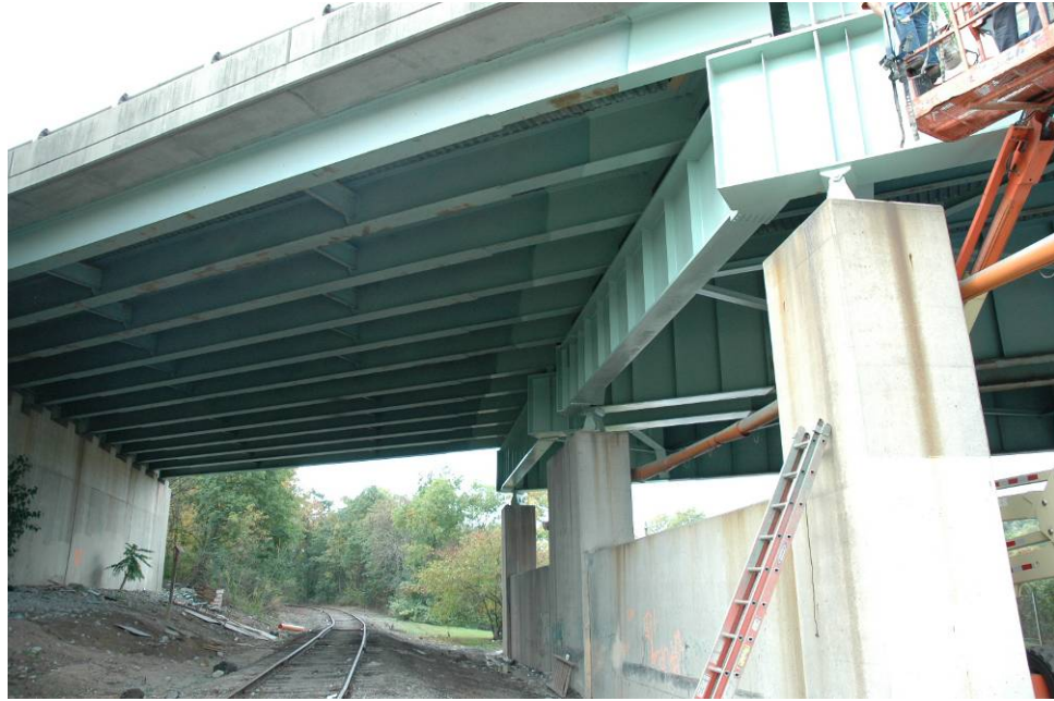
Figure 8 At Pier 1 cross girder connecting bracket projection from the main girders of Span 2.
