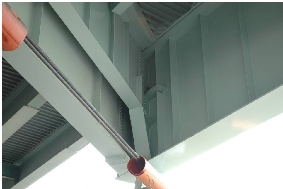
Figure 7 At Pier 1 girders connected by floor beam and cross girder parallel to the skew.
