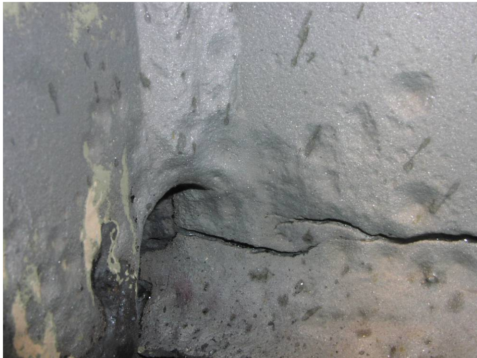
Figure 13 Crack origin (south side of bearing stiffener)
