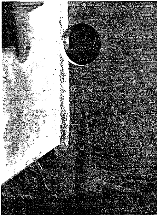
Figure 57: Retrofit hole (1 1/4 in.) at crack tip T4-I G12
