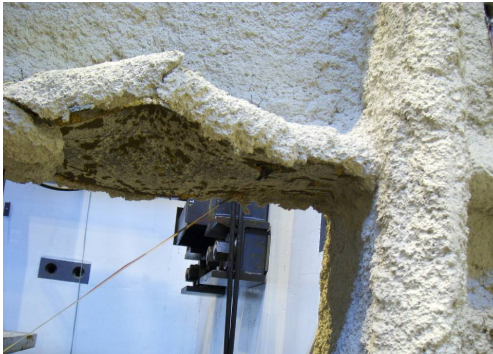
Figure 4.31 – Damage to SFRM during step 11 of WM assemblage test
