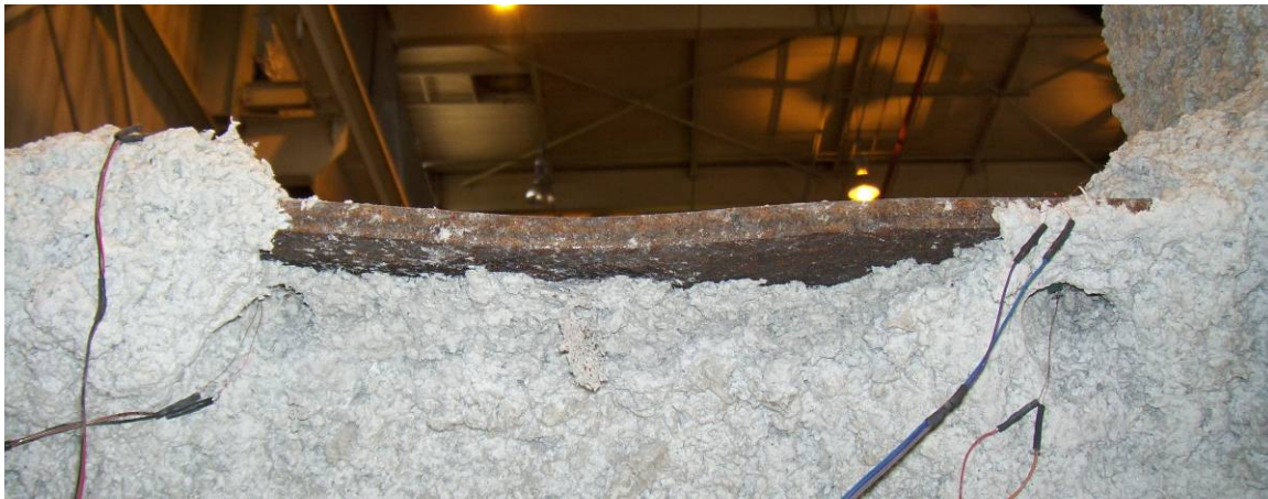
Figure 4.51 – Top flange of DM assemblage after loose SFRM was removed from underside of flange post-testing inspection
