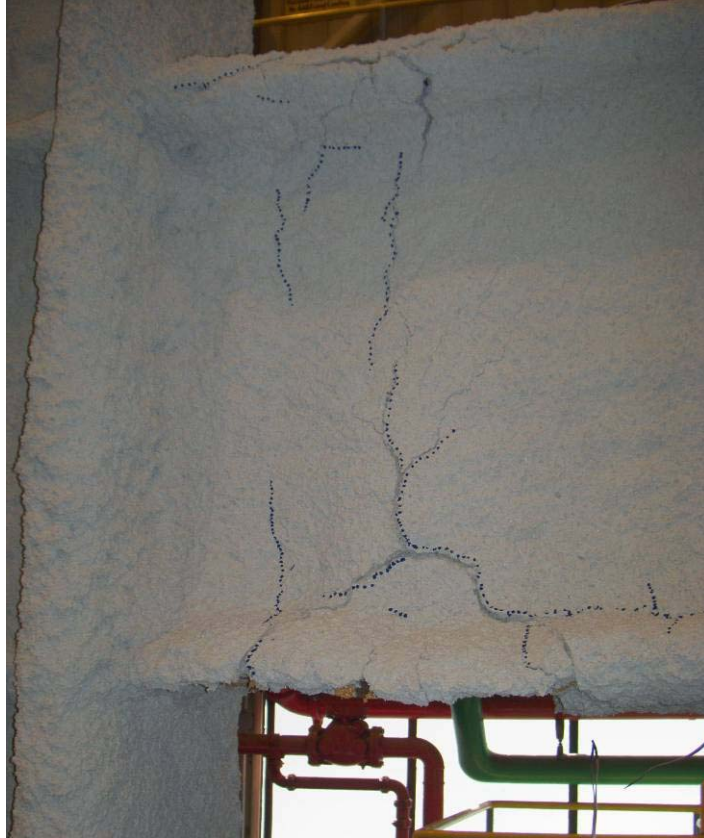
Figure 4.59 – Extensive cracking in SFRM of WM assemblage throughout web during post-testing inspection
