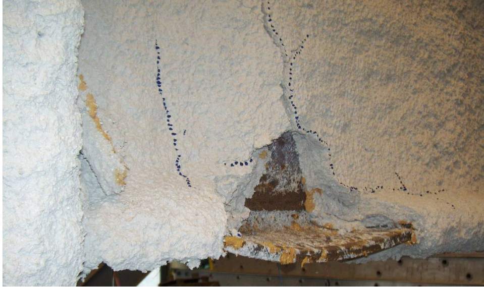
Figure 4.61 – Damage to SFRM on top of bottom flange, progressing into web of WM assemblage during post-testing inspection
