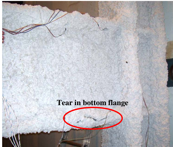
Figure 4.7 – Tear in bottom flange seen during step 10 of loading shown as Point A in Figure 4.6
