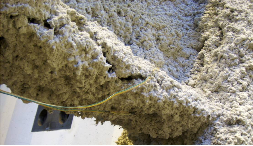
Figure 4.52 – Close-up view of longitudinal splitting in bottom flange SFRM of DM assemblage during step 10
