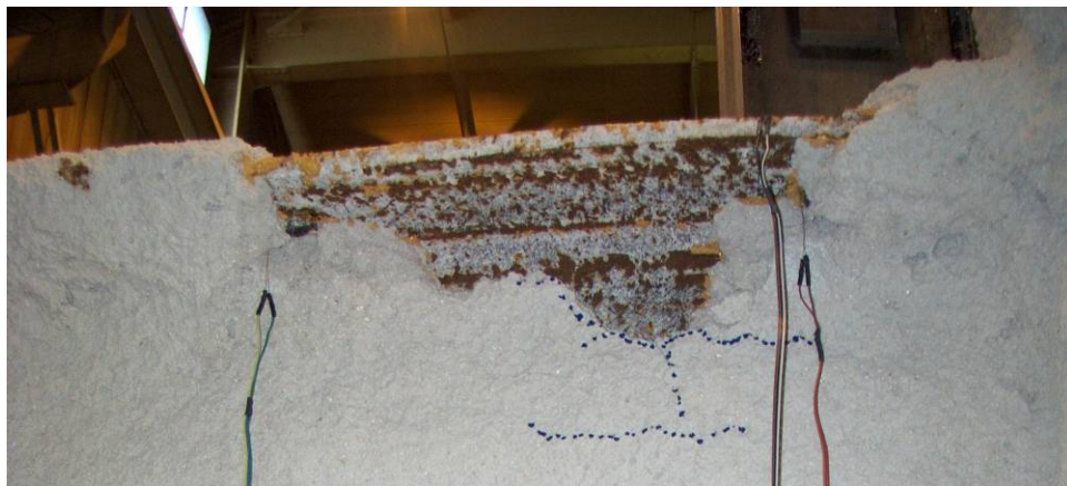
Figure 4.60 – Damage to SFRM on bottom of top flange, progressing into web of WM assemblage during post-testing inspection
