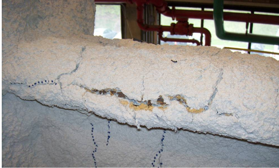
Figure 4.57 – Extensive cracking of SFRM on top flange of WM assemblage during post-testing inspection
