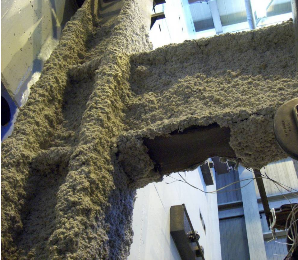
Figure 4.53 – First damaged portion of SFRM on bottom flange of DM assemblage during step 10
